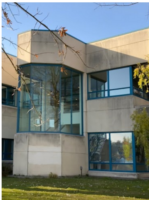
Hazardous see-through conditions and reflections at the Marine Studies Building on the UW campus.
